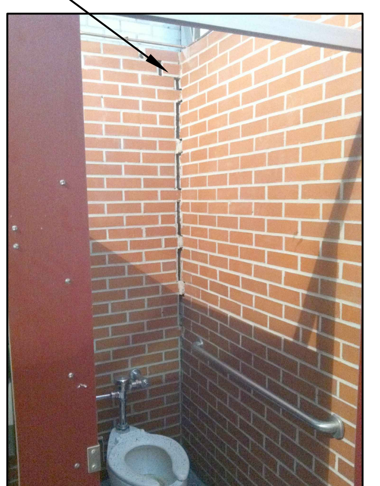
2b MASONRY WALL SEPARATING AT CORNER OF GROUND LEVEL WOMEN'S RESTROOM #4
